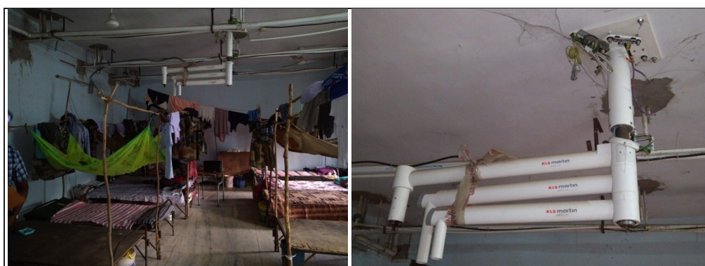
Photograph taken on 04 October 2019 showing proposed Operation Theatre of the Dental Institute and incomplete installation of OT Light.
